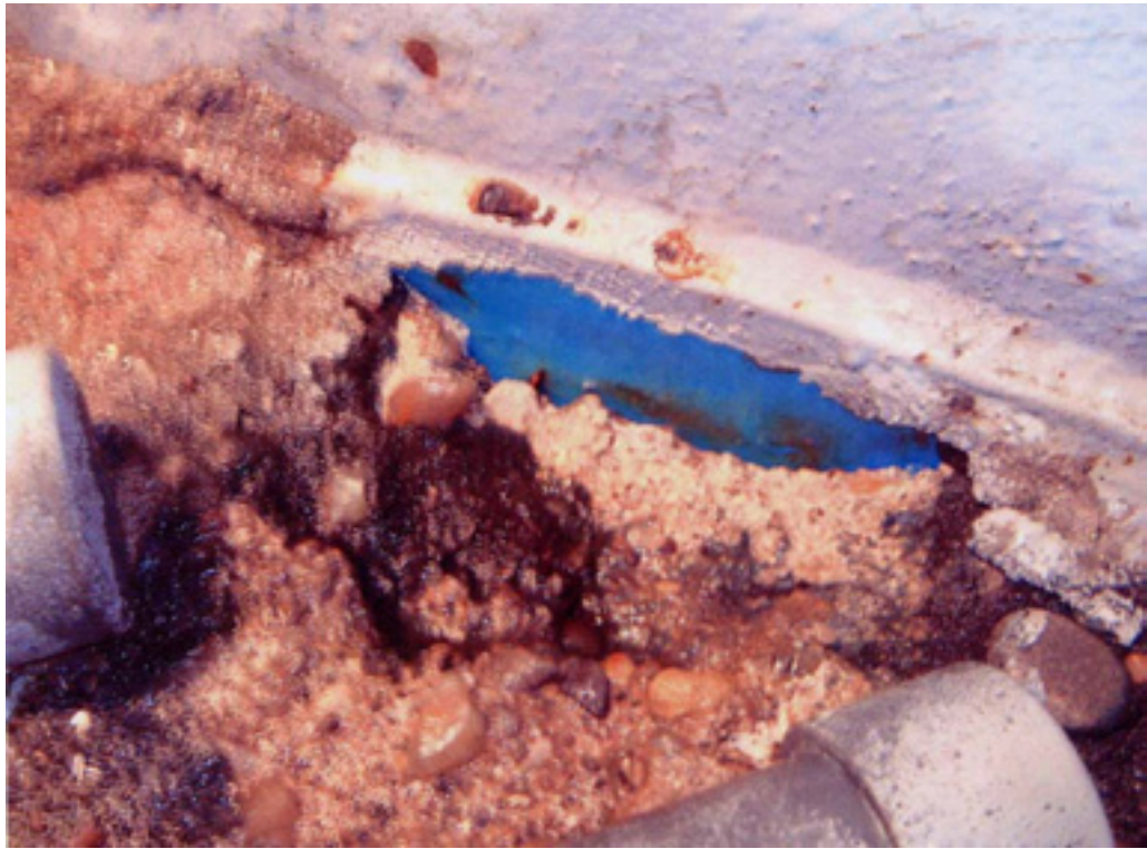
Figure 15: Filter C, Deterioration of concrete against filter container face
