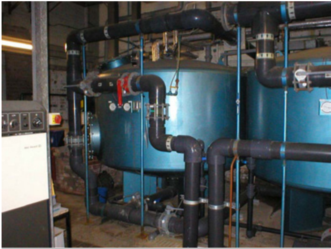
Figure 8: Filter C, one of two filters processing the water of the large pool.
