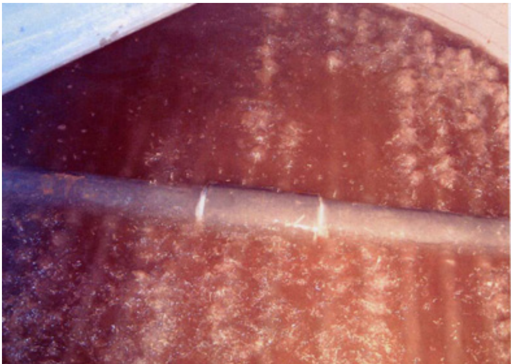
Figure 9: Filter C, Air scour pattern very poor
