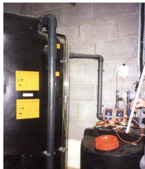
Sodium hypochlorite bulk and day tanks
