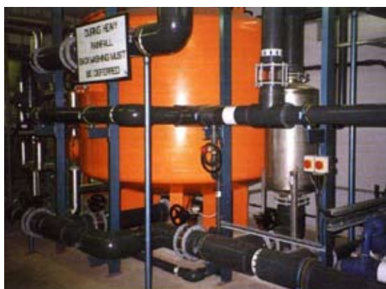
Ozone contact vessel and de-ozone vessel
