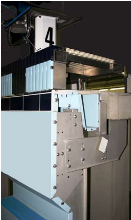
Tank under construction in stainless steel panels with an integrated overflow and raised end
