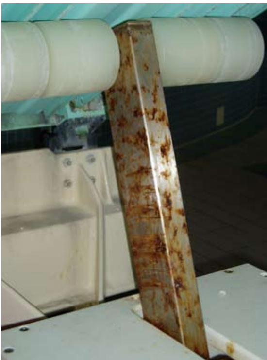
Corrosion to stainless steel fittings
