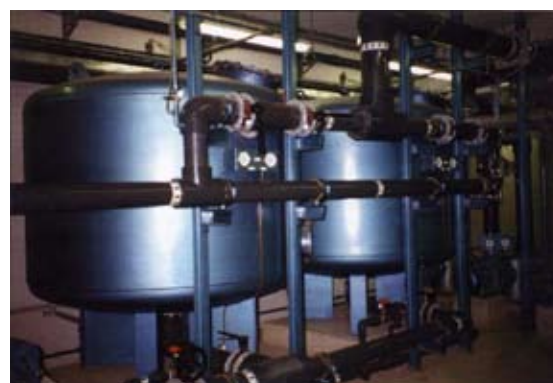
Typical filter installation
