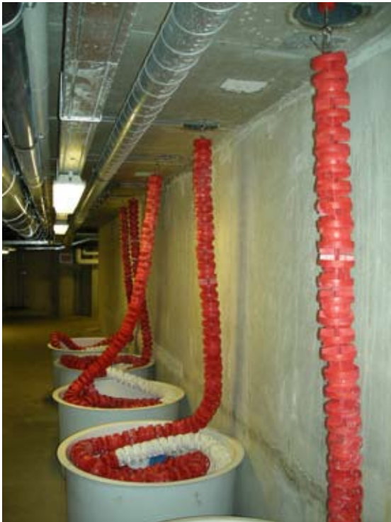
An alternative to storing lane ropes in a Pool Store – lane ropes can be stored in hoppers in the pool undercroft and accessed through stainless steel covers set into the pool end surround
