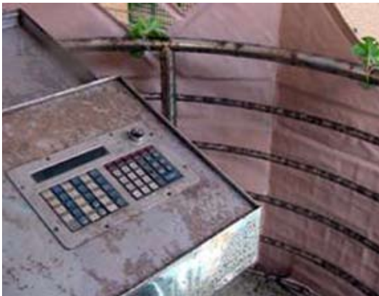
Corrosion of stainless steel balustrading and control panel exposed to pool atmosphere
