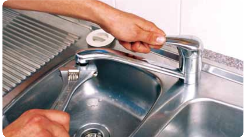
Install flow restrictors on all non-regulated fixtures and repair or replace them as part of an active maintenance program
