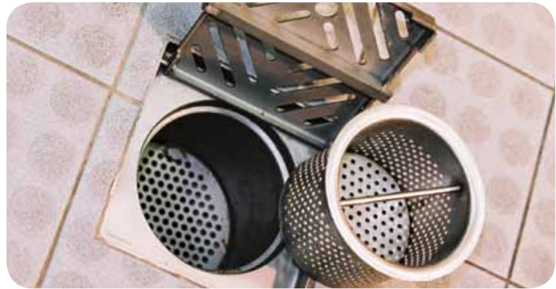
In-floor bucket traps capture food scraps, cutlery and cleaning cloths that may have fallen on the floor. They prevent these items from entering the grease arrestor and encourage thorough cleaning practices
