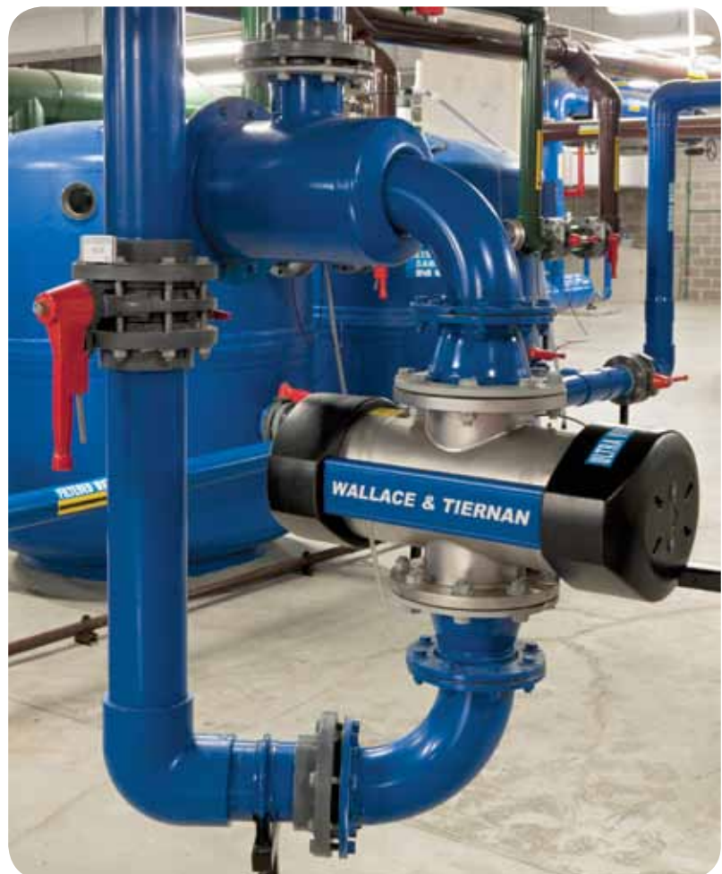
UV systems like this one at Ian Thorpe Aquatic Centre effectively disinfect and sanitise water
