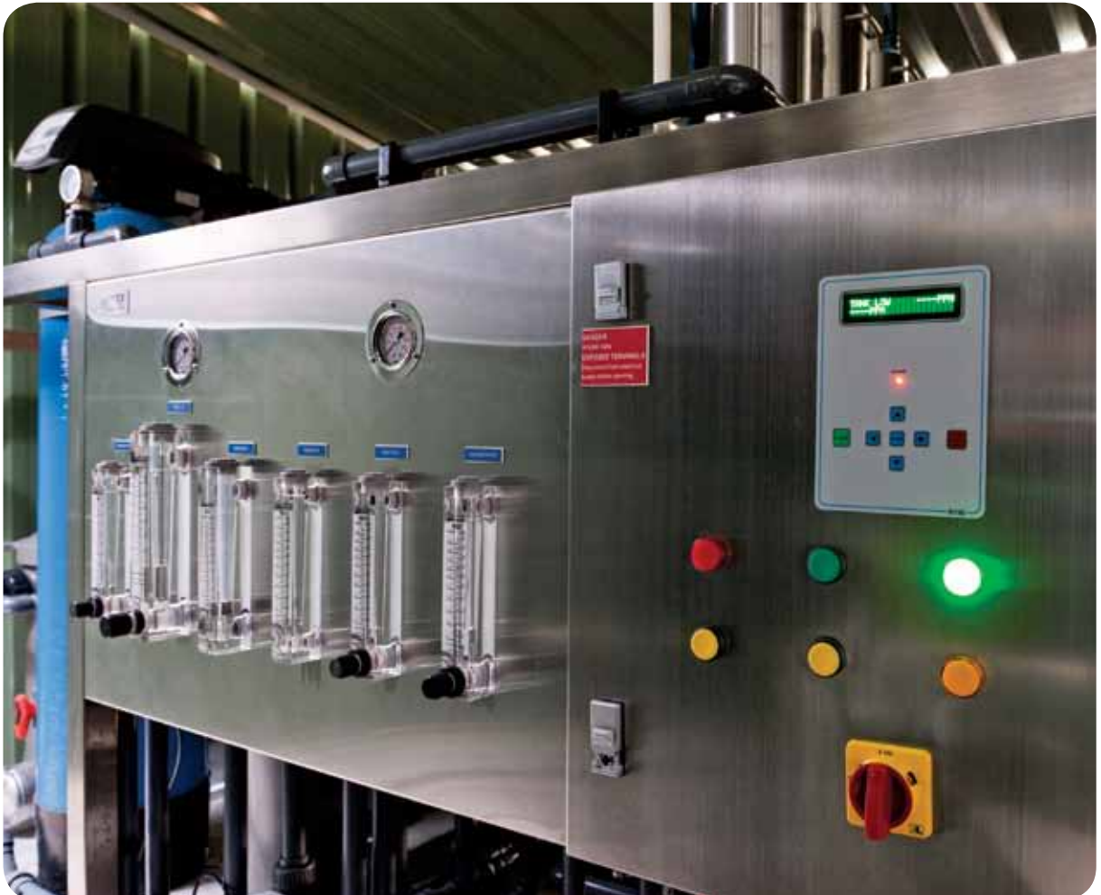
Minimise your water use before considering recycling systems, like this backwash water recycling system at Warringah Aquatic Centre.
