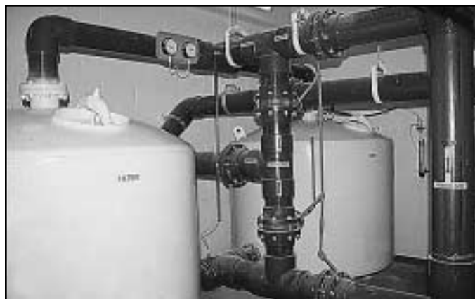
Sand filter system.
