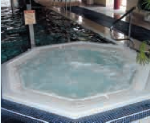
Commercial spa pool
