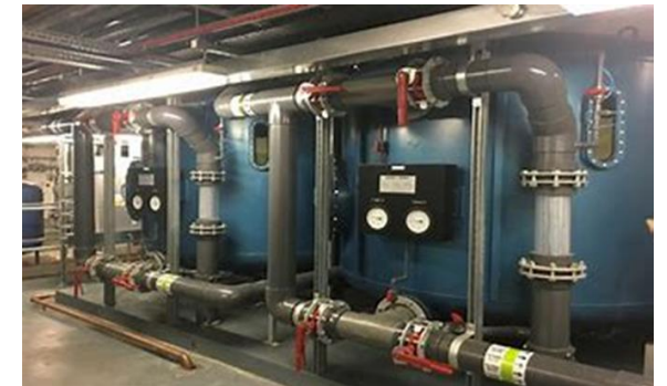
Multi-grade sand filter
